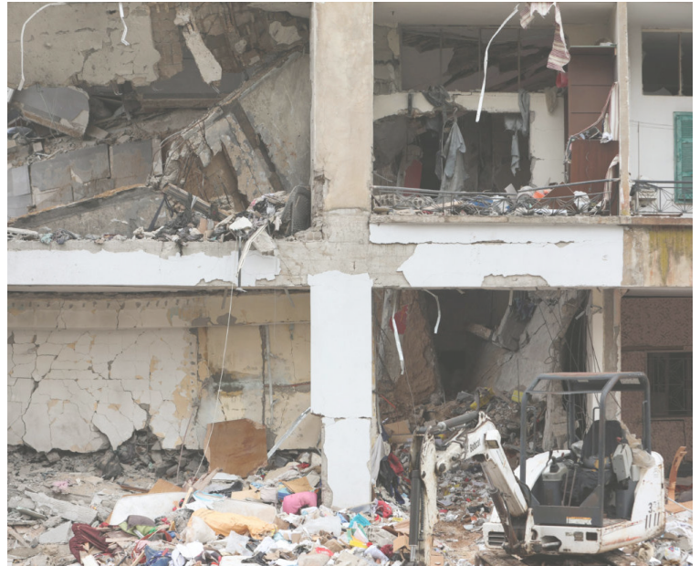
A view shows a damaged building after what security sources said was an Israeli strike in Nabatieh, southern Lebanon, Feb. 15, 2024. (Photo: Reuters/Aziz Taher)
